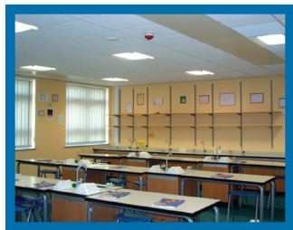
Ceiling radiant panels.
