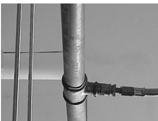
Figure 4: Chilled water pipe with slight condensation visible after opening windows.
